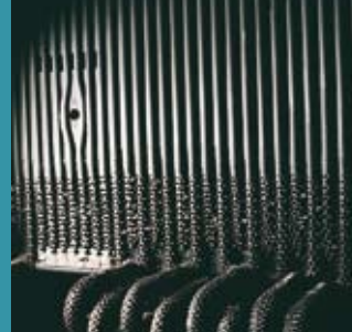
Boiler tubes district heating station can withstand temperature cycling, corrosive environments and fluctuating particulate levels.
